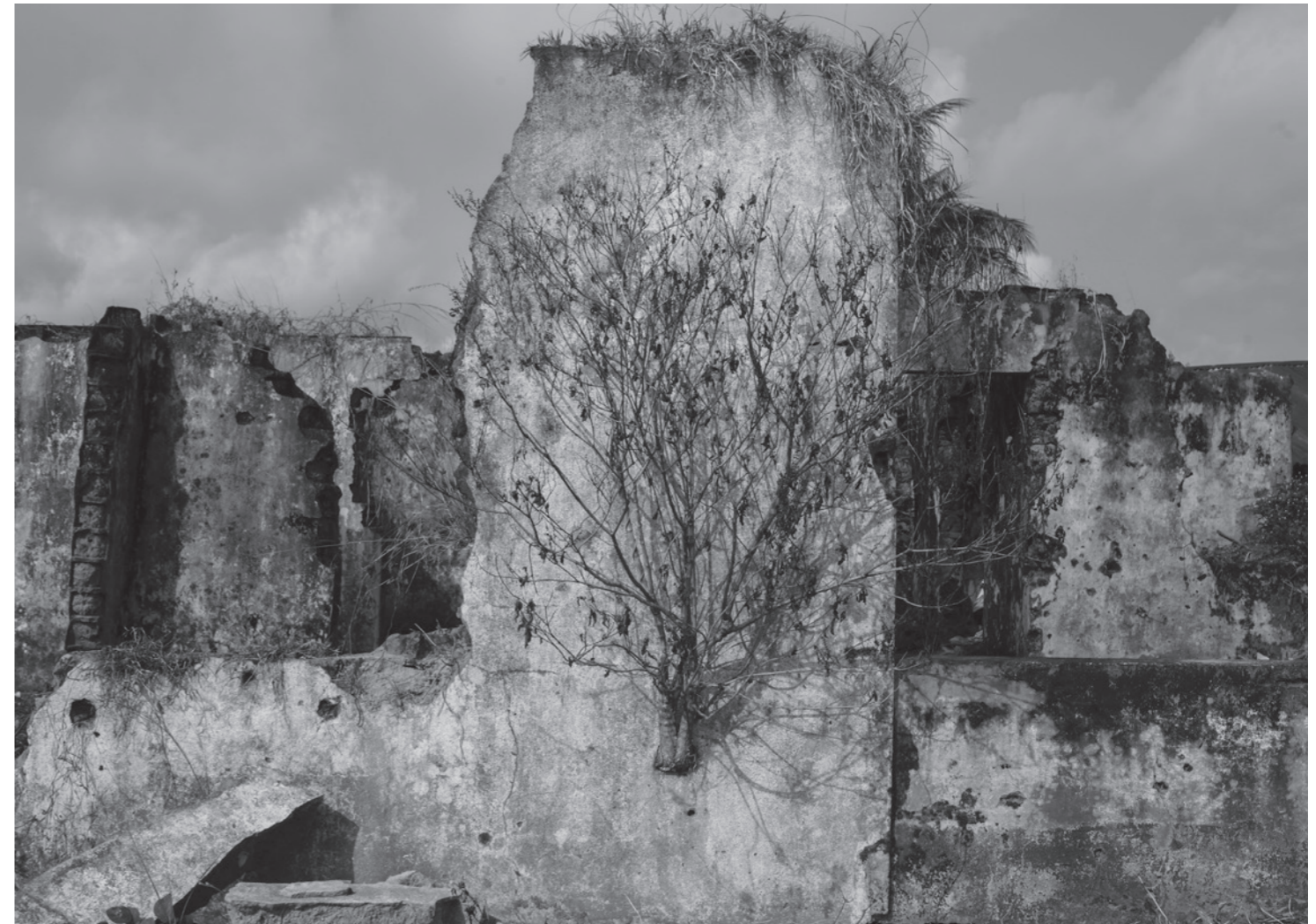
A tree growing through an abandoned house, Liberia, February 2018.
